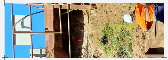
The hopper at the top of the slope, linked by pipe to the waste oil storage tank.
